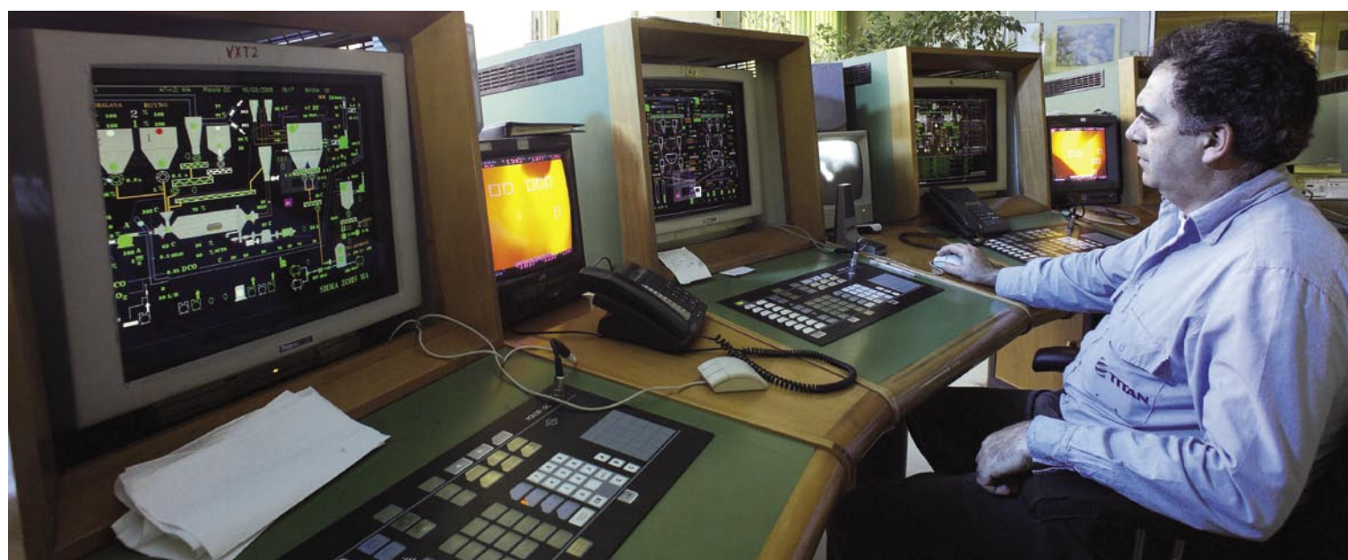
Control panels, Patras plant, Greece
