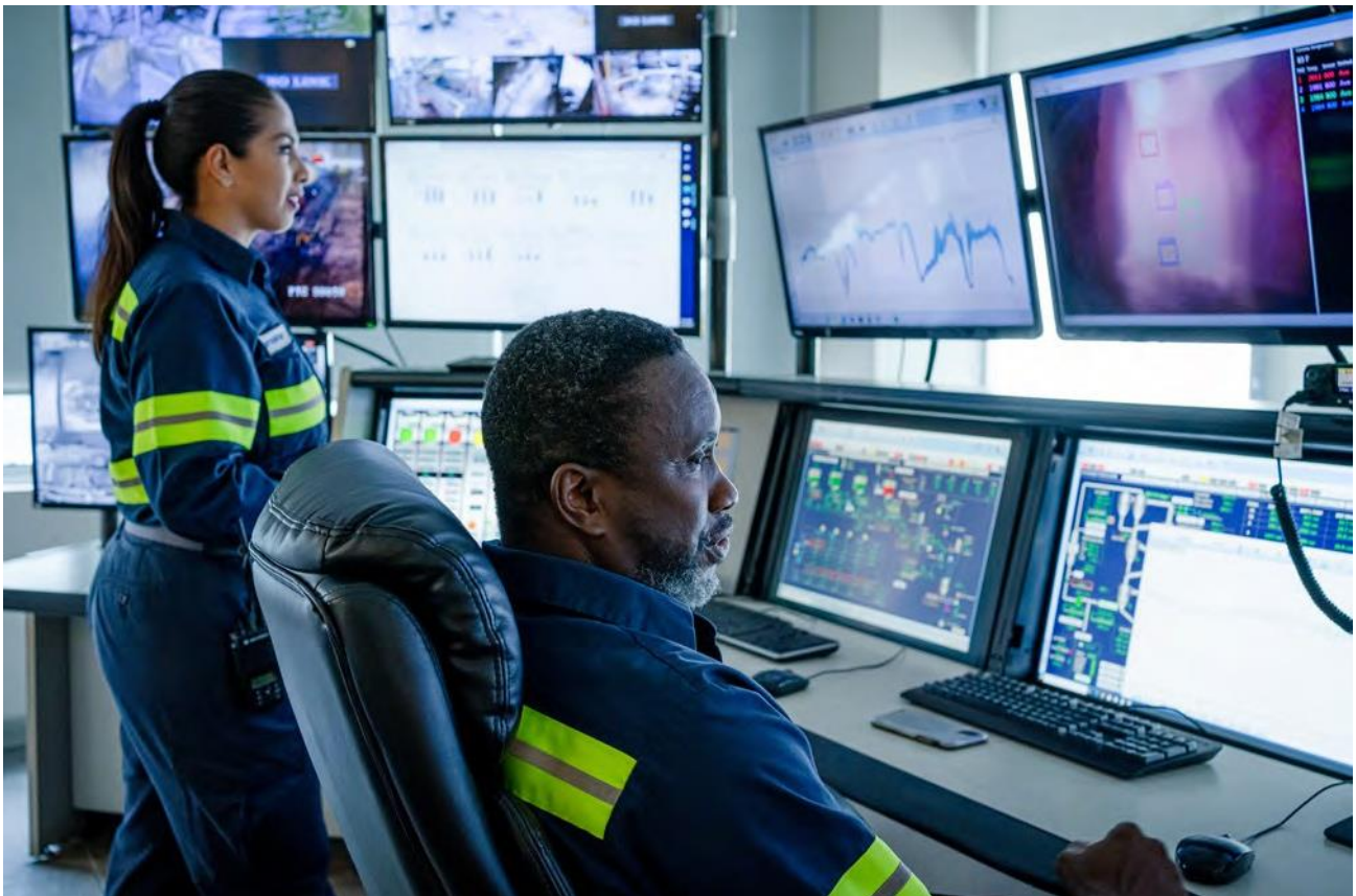
Control room at Pennsuco cement plant, USA
