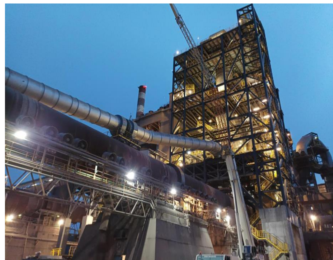
Kamari Kiln Line #1 Calciner
